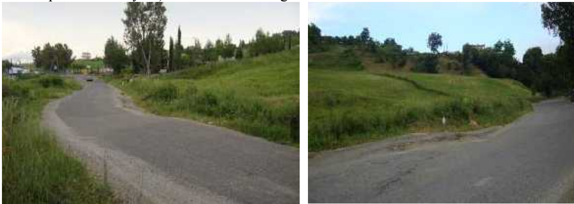
Figure 1. Photos from the existing road landslide.
